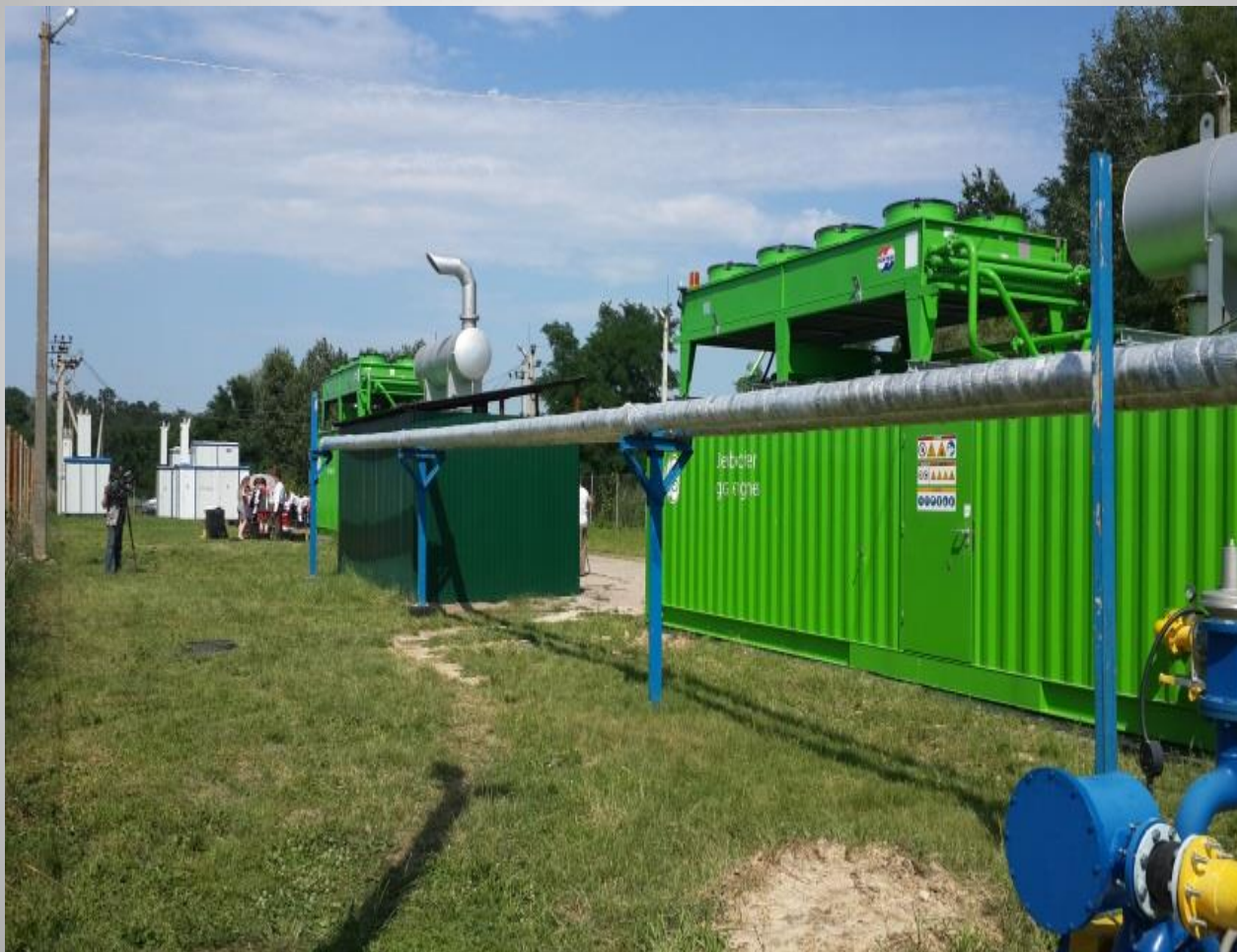
Landfill gas. “LNK” Ltd., Cogeneration at five sites
