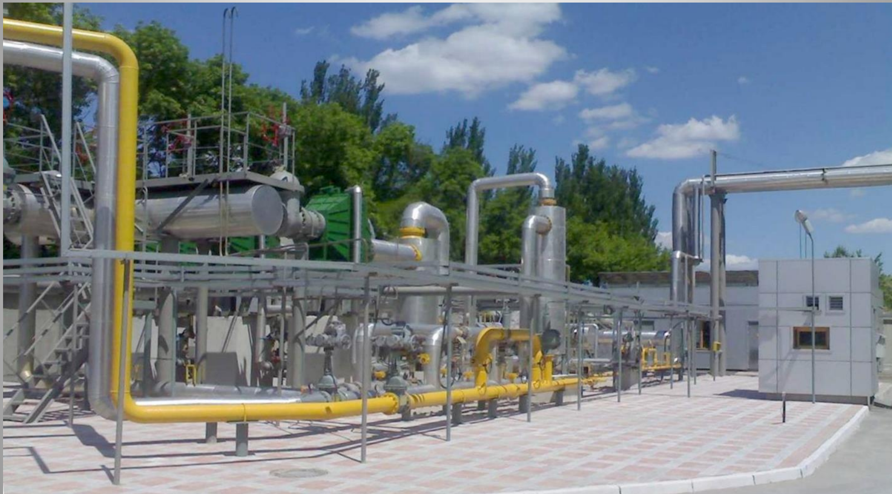
Zasyadko Coalmine, coalmine methane, 72,7MWel.
