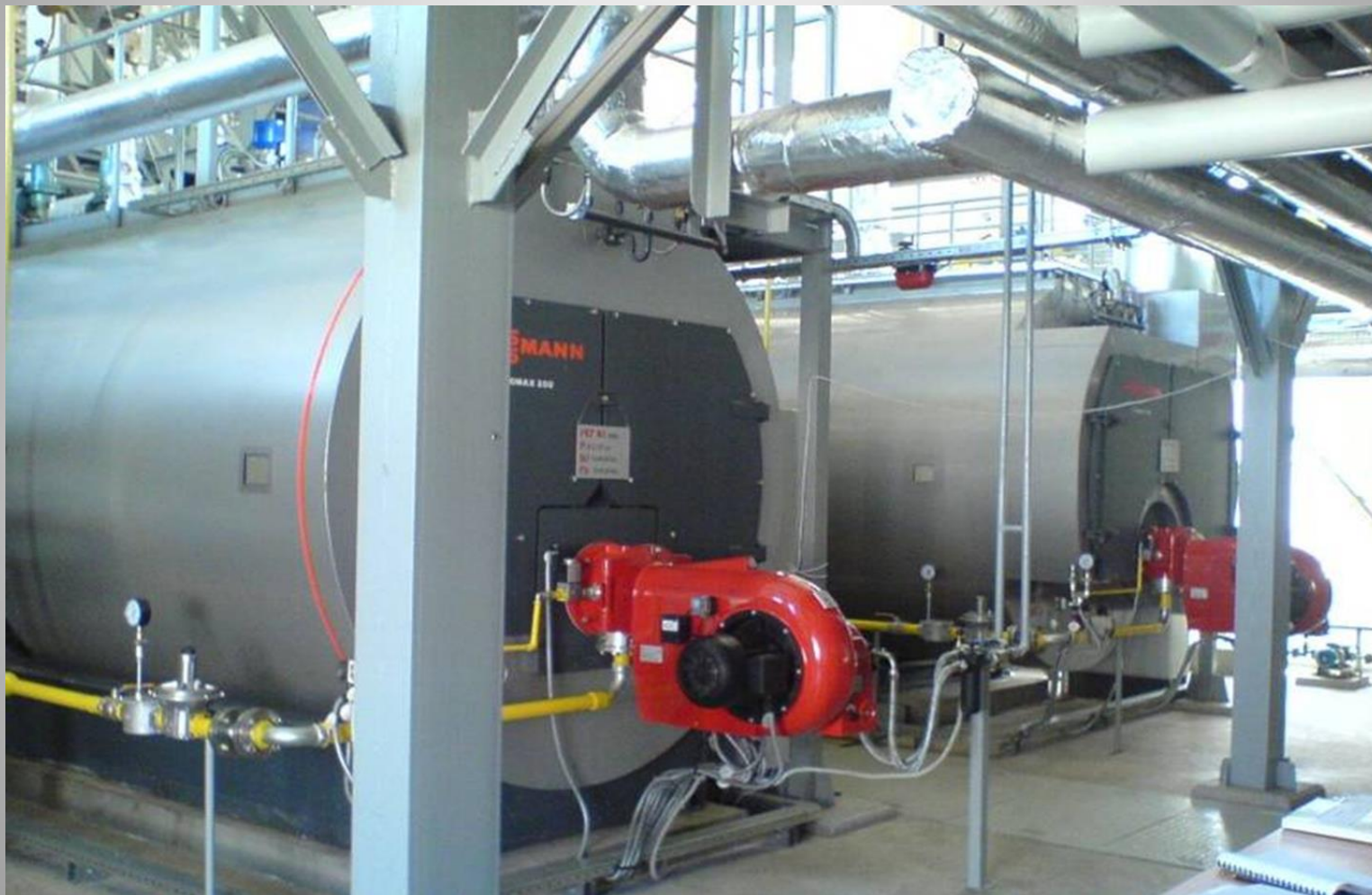
National Bank of Ukraine, Banknote Paper Plant, 2.1 Mw eI
