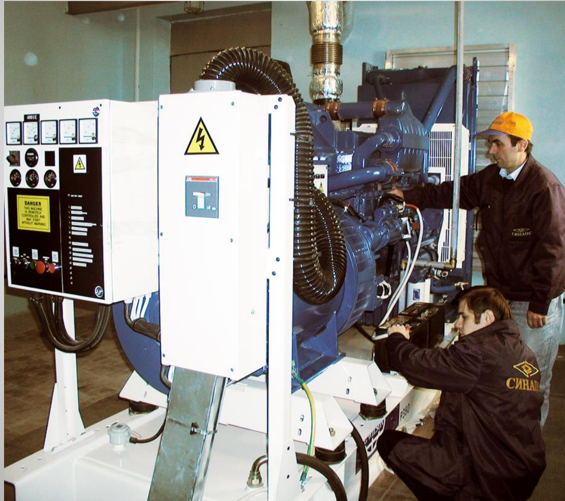
Diesel Equipment Maintenance
