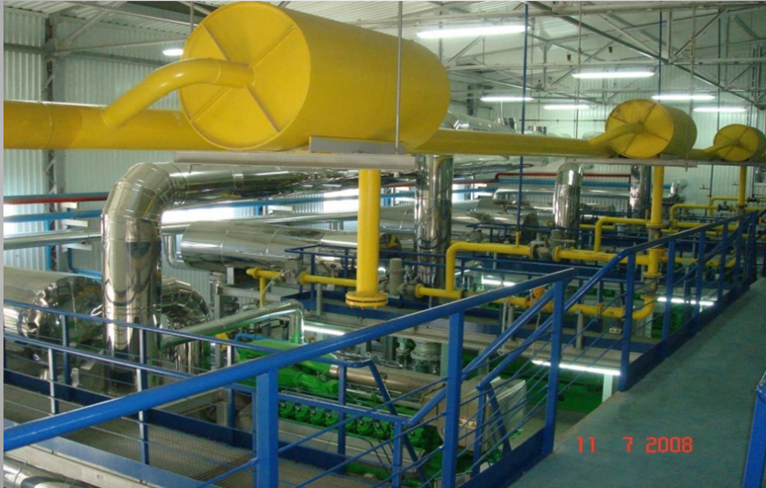
Illichevsk Fat and Oil Refinery Plant, 5,7 MW el
