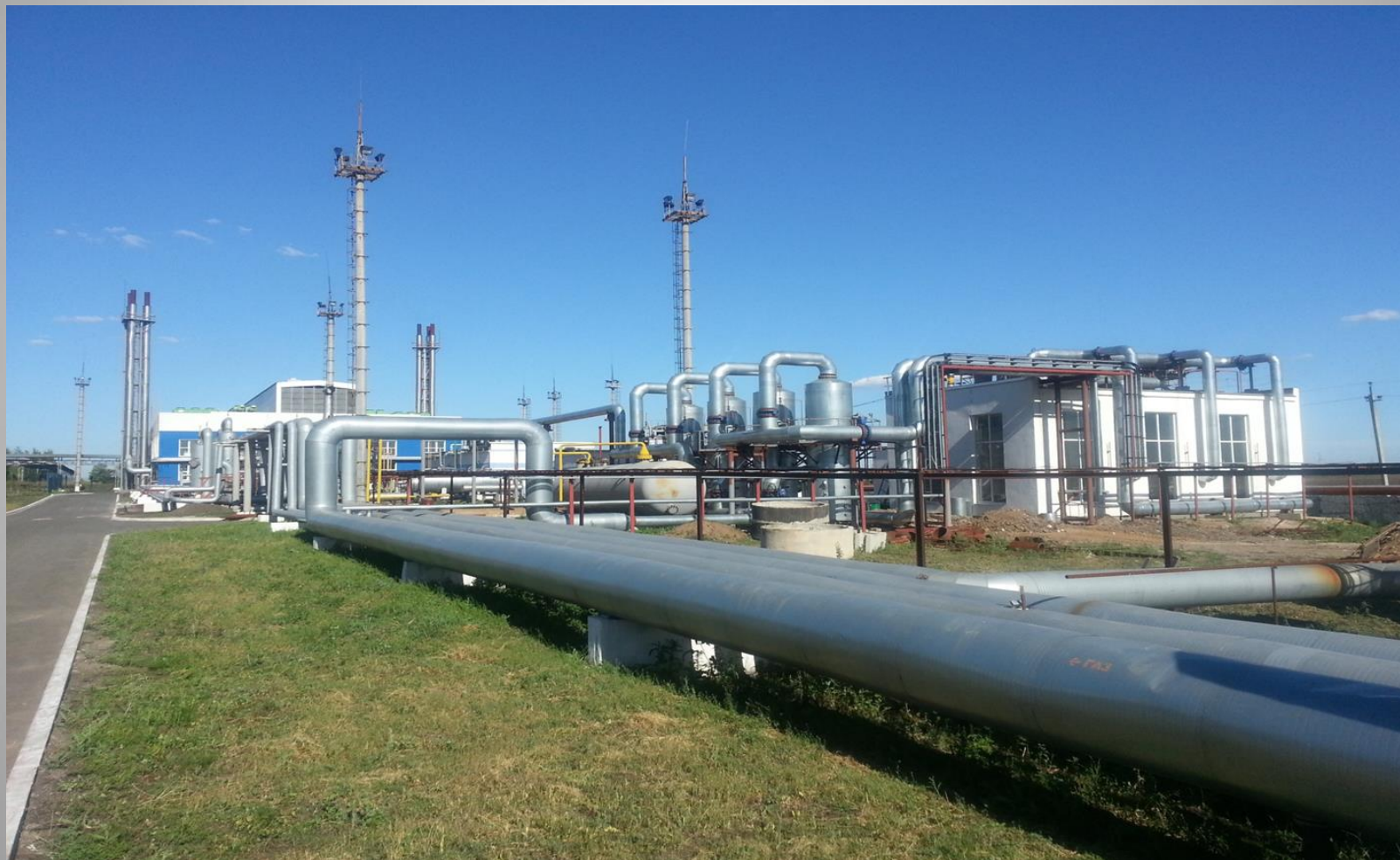
Coalmine “Pokrovskaya”, 75 MW el
